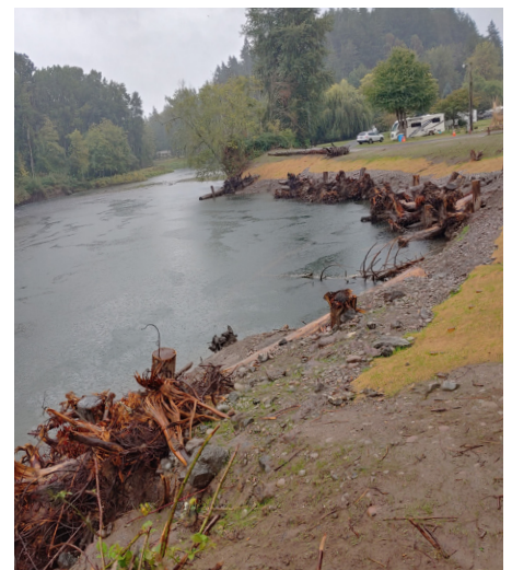
Photos: River bank at Camp Kalama pre-project (top) and at the same project site after Cowlitz Conservation District began taking action to stabilize the riverbank (bottom).
