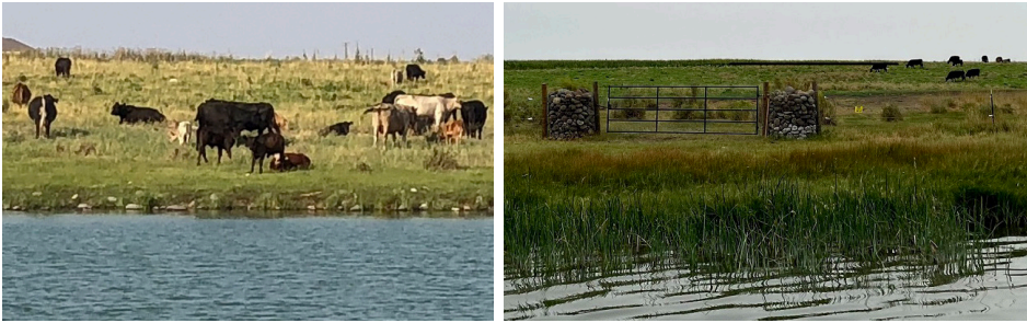
Grant County Conservation District used LTA to help an operation where livestock had uncontrolled access to a shoreline area (left). The district installed livestock exclusion fencing, rock cribs, and a gate for maintenance and landowner access (right).
