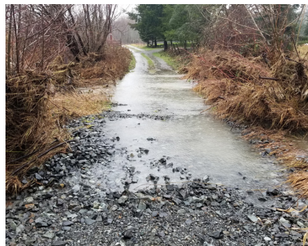
This private road's culvert exacerbates flooding of Haystack Creek and presents a barrier to Chinook and Steelhead trout. (photo by Snohomish Conservation District)
