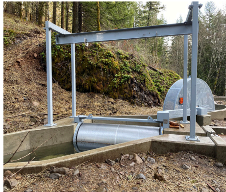
New rotary drum fish screen, constructed by the Washington Department of Fish and Wildlife and installed in 2019 for White Salmon Irrigation District. (photo by Carly Lemon)
