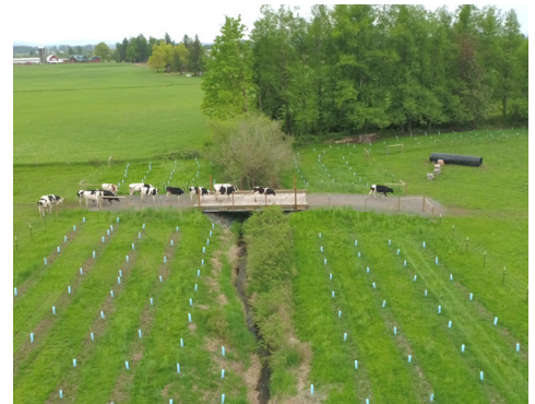
Culvert to Bridge along Kamm Creek. A local farming group documented this story featured here: https://youtu.be/hxViMuXzJIU . (photo by Veritas Media)
