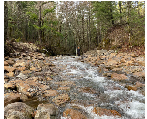
Constructed channel in Buck Creek, designed to provide fish passage over the old diversion dam. (photo by Carly Lemon)
