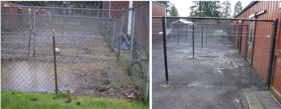
LTA helps conservation districts start a relationship and develop conservation plans with landowners. Often this leads to project construction, such as this example from Kitsap Conservation District that shows a site before (left) and after (right) the district helped harden surfaces and upgrade fencing.
