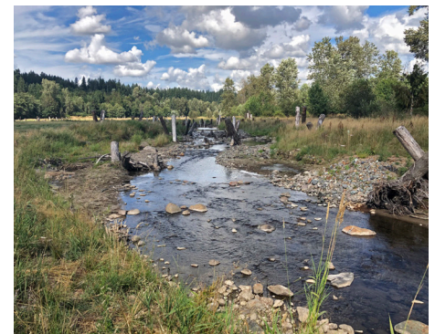
The new side channel and large woody debris installed at South Prairie Creek Preserve.
